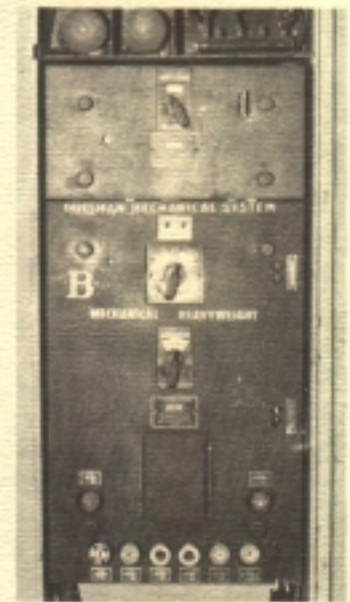
Air conditioning system control panel, located near porter's seat on Glengyle. (Photo by J. W. Schroeter)
