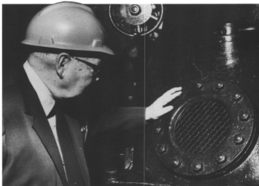
Former Holtwood superintendent W. Roger Small Jr. checks the glass inspection port on the Unit 5 thrust deck that enables operators to view the oil-bathed bearing during operation.
